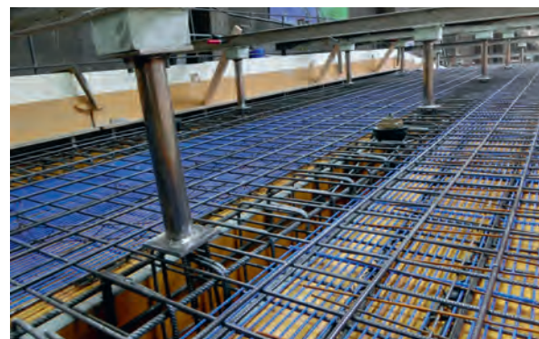
03 Position of the capillary-like piping system in the prefabricated reinforced concrete part beneath the outermost reinforcement layer, shortly before pouring the concrete.
